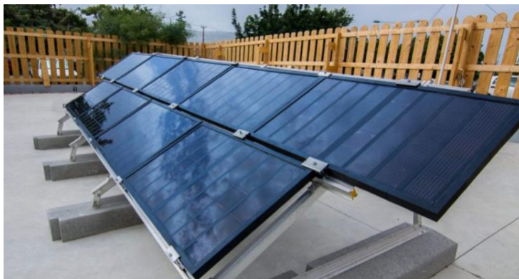
Figure 1: A photograph of the solar farm
